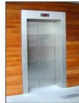
Passenger Elevator Auto
