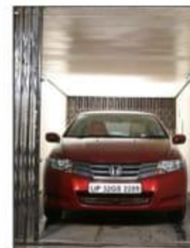
Freight / Car Elevator
